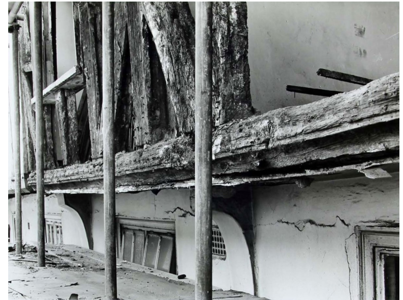
Fig. 5.21 July 1965 photo showing the restoration of the second floor framing to the front of no.89 © Historic England.
