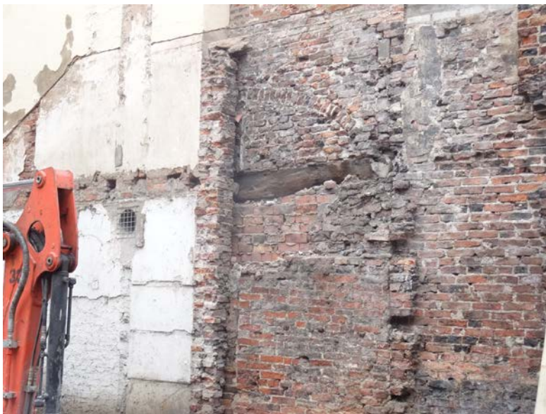
Fig 2. – Condition of newly exposed party walls – several areas of defective masonry.
