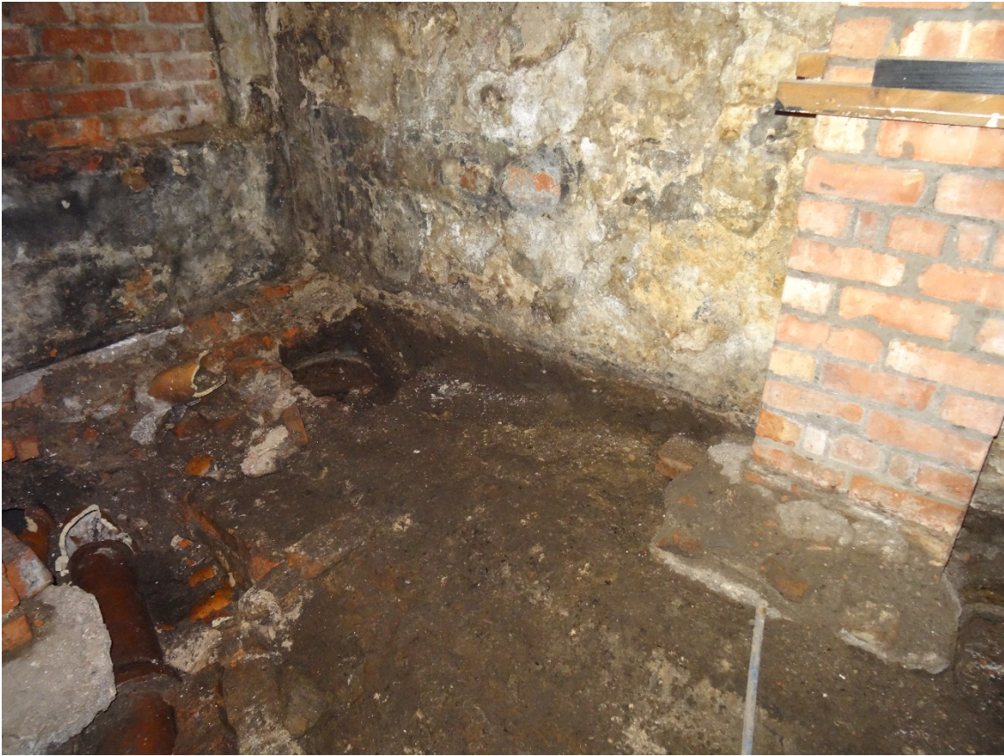
Fig 5. Basement walls founded on earth with inadequate foundations.
