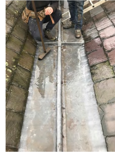
MAINTENANCE Example of valley gutter cleaning at York Theatre Royal, this needs to be undertaken on a 3-month cycle.
