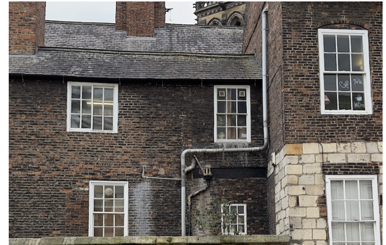
Figure 15 Existing External Foul Pipework on the south-west elevation (from St Leonard's Place).
