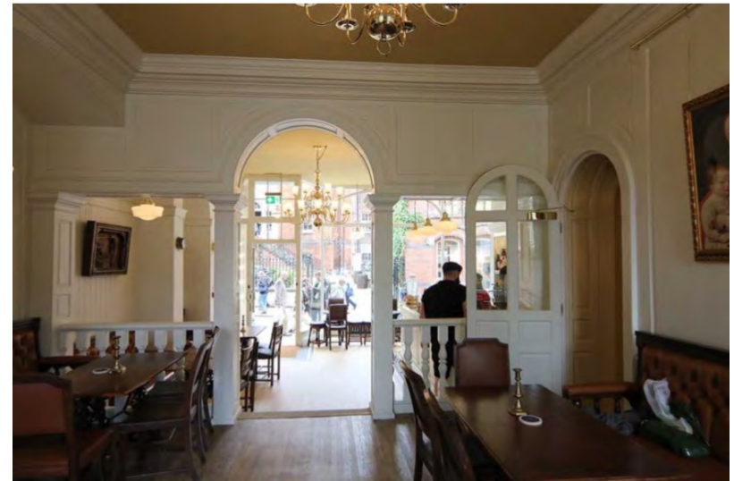
RESTORATION Archway restored to ground floor of 14 Lendal. New timberwork made to exactly replicate the original fabric by tracing their outline in the original paintwork
