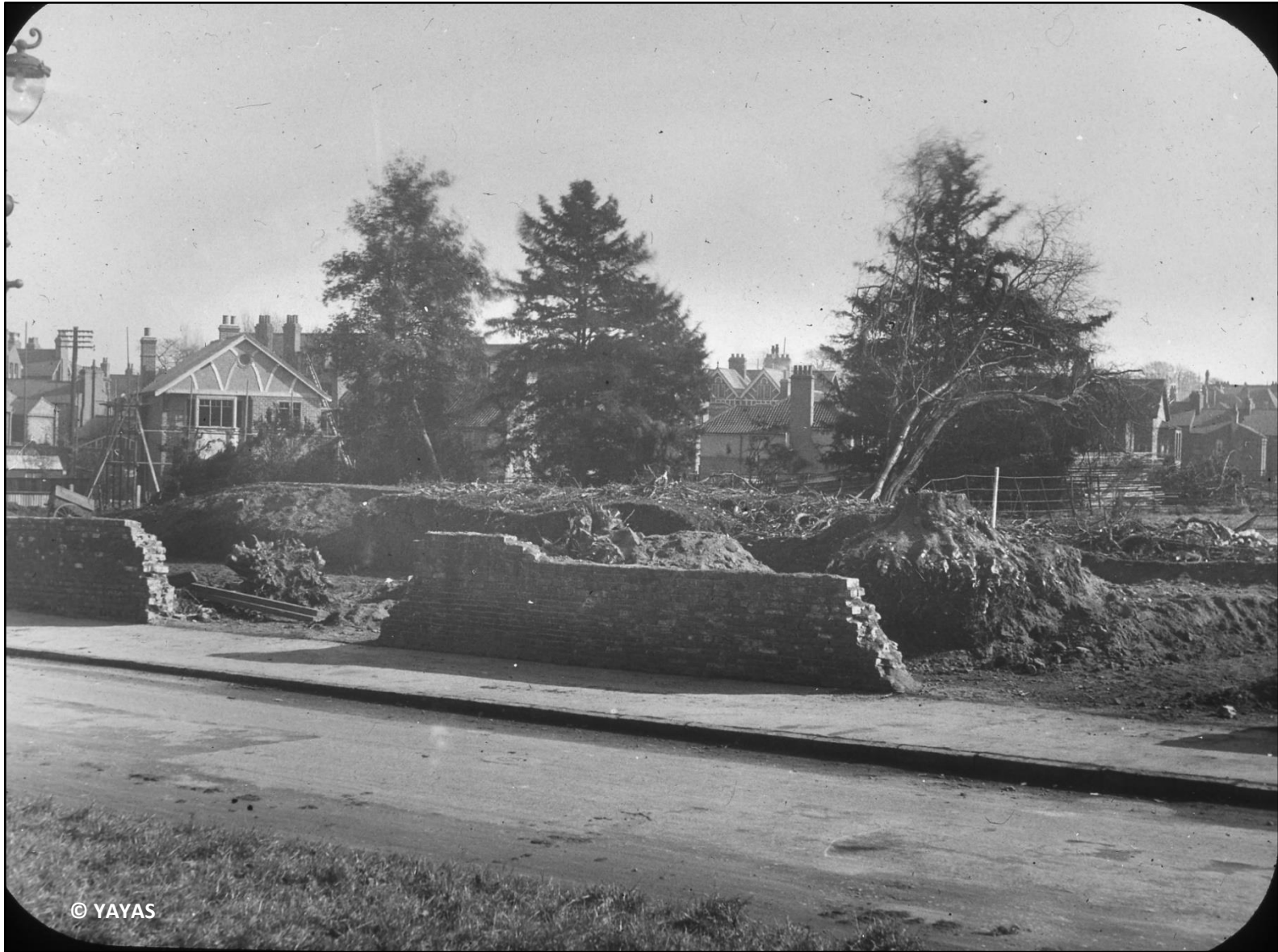
Figure 77. The former Clifton Croft complex from Water End, likely 1931-1932. The boundary wall of the complex can be seen partially demolished. No. 1 Greencliffe Drive can also be seen with its distinctive gable end on the left-hand side of the photograph (YAYAS EV2758).
