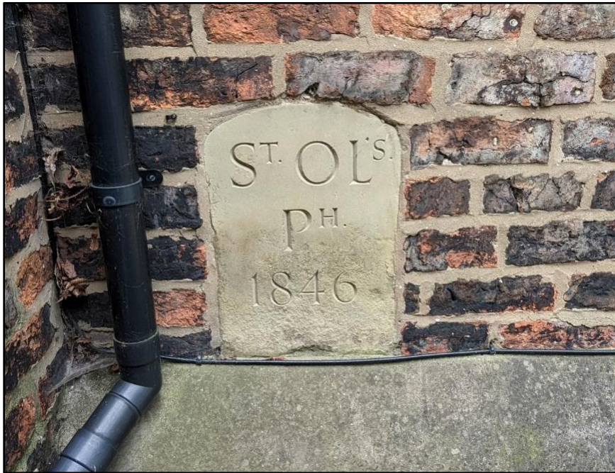
Figure 52. Date stone as seen on the southern elevation of No. 16 Clifton Green, built as a Gardener's House for John Roper the younger around 1846. The house lies on the boundary of St Olave's Parish, as indicated. Spring 2023.
