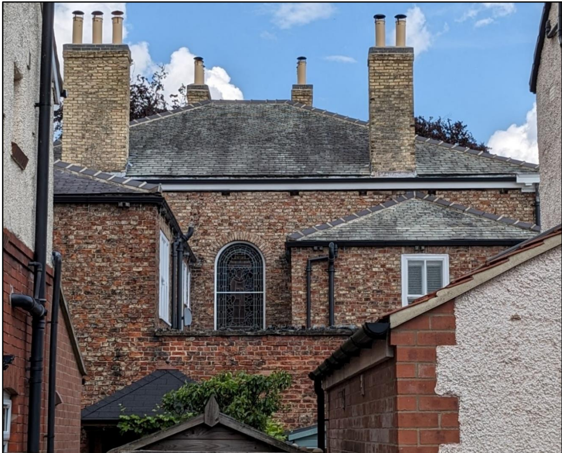
Figure 38. The rear of Clifton Croft as seen from between Nos. 13 and 15 Westminster Road. The building's incorporation into the boundary wall and stained-glass stairwell window can be seen. Summer 2023.
