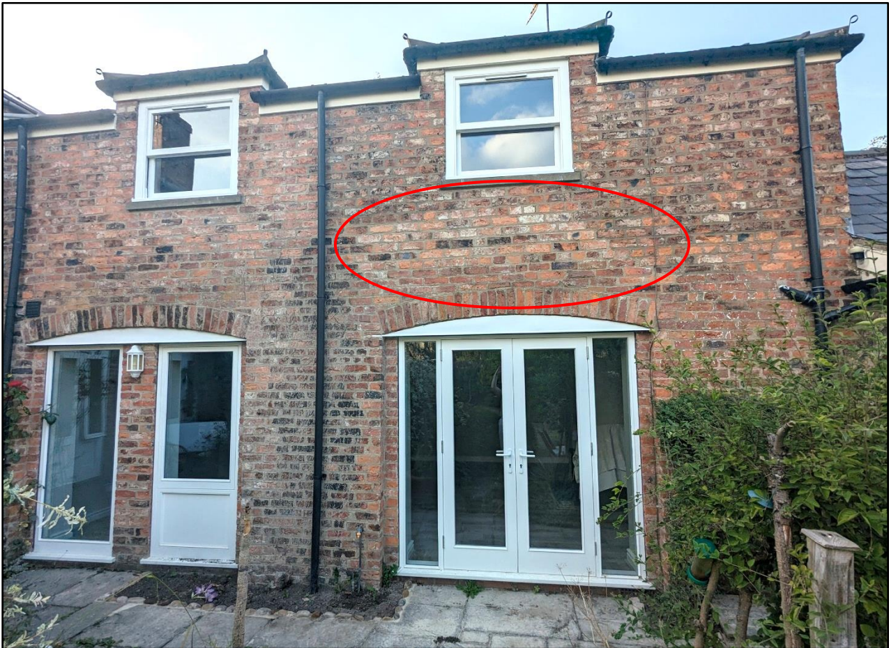
Figure 48. The two-storey portion of No. 3 The Mews is shorter than Nos. 1 and 2, with dormers around the first-floor windows. The doorways into this part of the Stable Block are also lower than the doorways of Nos. 1 and 2. The brick scar from the former attached single-storey extension can be seen, circled in red. Summer of 2023.
