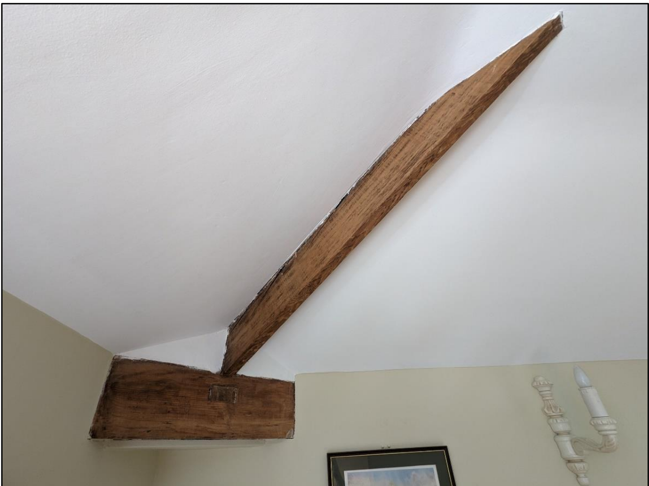
Figure 47. Wood beams like this one shown are present throughout the first-floor ceiling of No. 3 The Mews, with the building being lower in height than Nos. 1 and 2. Spring 2023.
