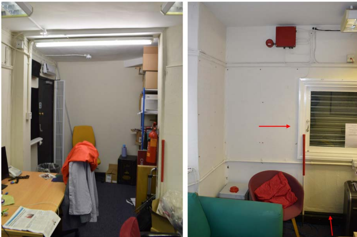
Figure 7: Left: Looking north, the original north wall has been removed to extend the room removing evidence of a window. Right: Looking west, the original doorway has been obscured by the insertion of a later window (Author 2022).
