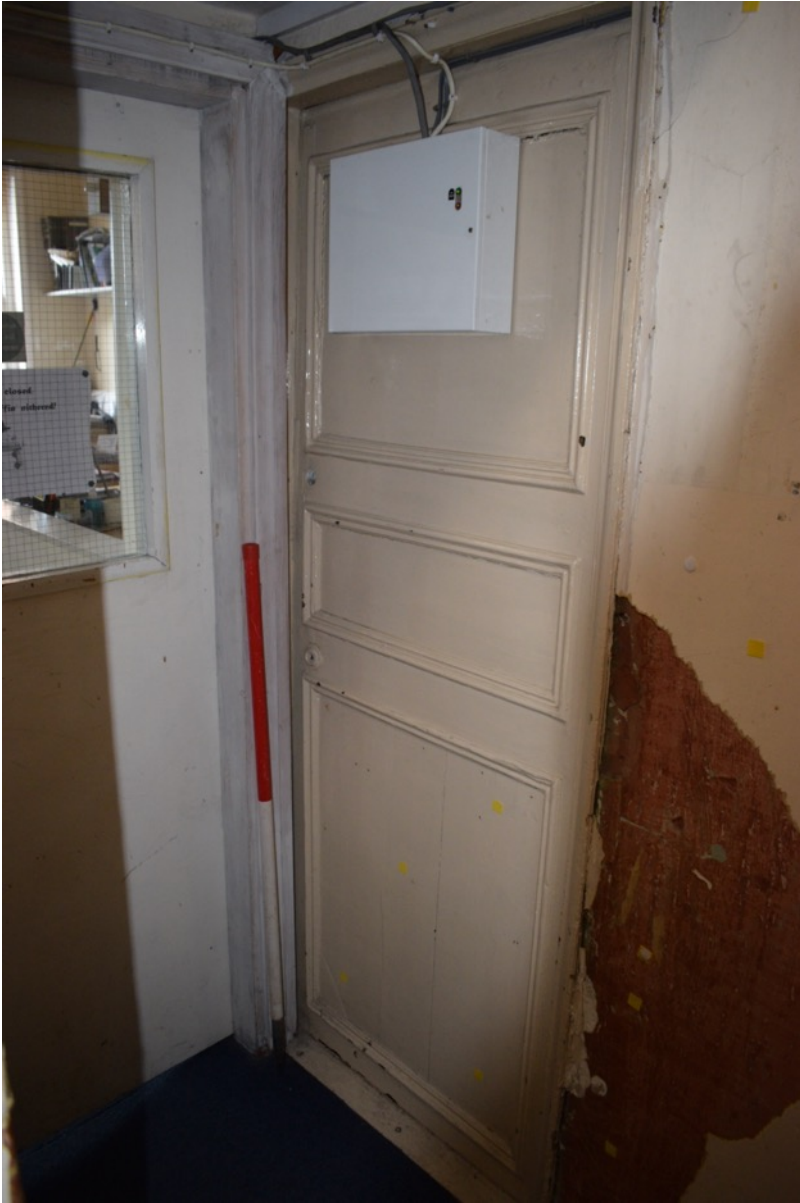
Figure 103: 2 nd floor landing looking west. Original 18 th century door that would have led to the small western room. This room no longer exists, and this door is not utilised (Author 2022).
