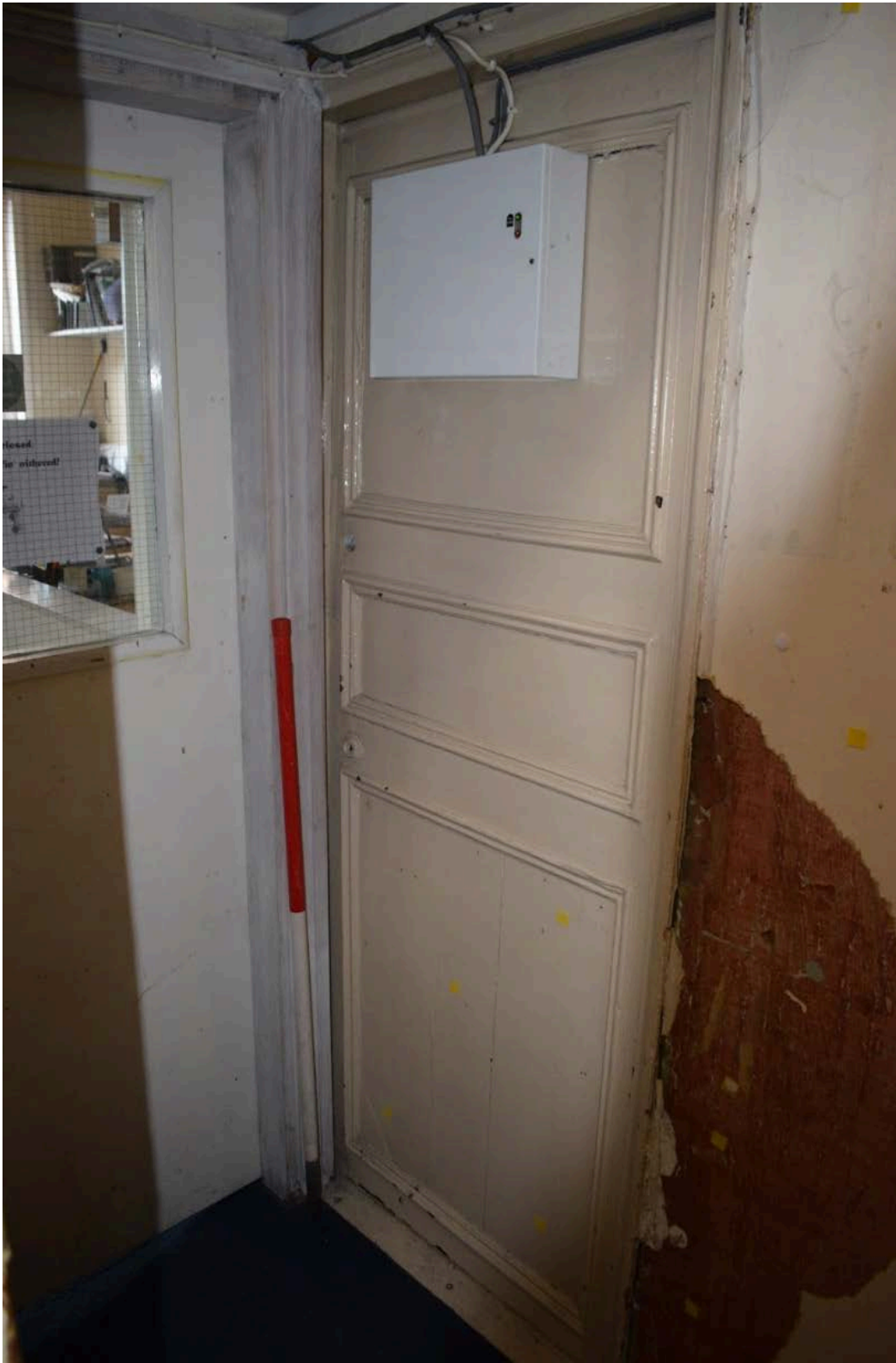
Figure 29: West wall of 2 nd floor landing showing door to Room 46. Room 46 no longer remains, and this door is no longer utilised (Author 2022).
