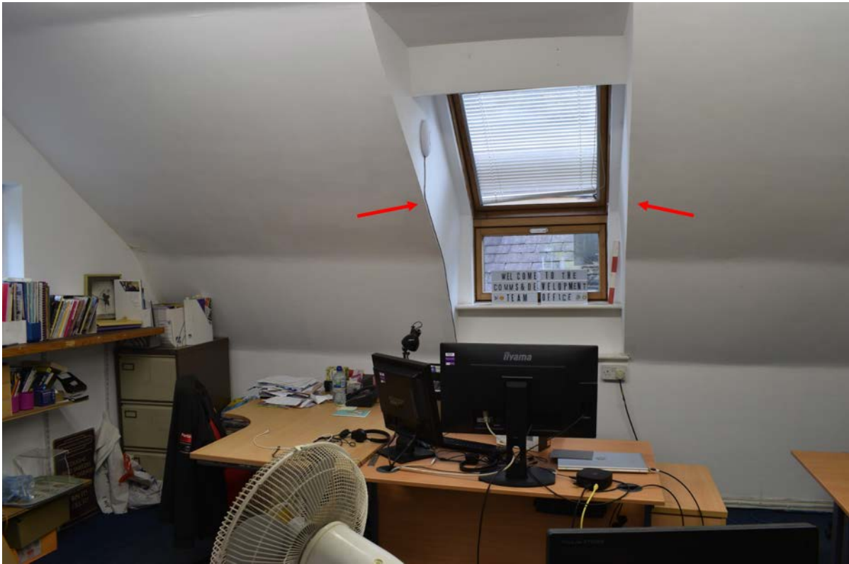
Figure 27: East wall of rear bedroom. Arrows show where a partition was present enclosing the space where the dormer is into a void. This divided the room into a front and back space (Author 2022).
