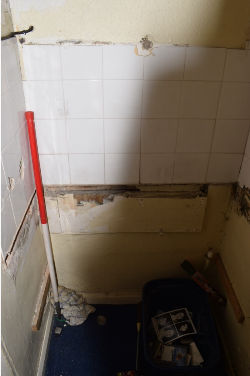
Figure 95: North-west anteroom off 1 st floor rear room facing south. This room was originally part of the 18 th century theatre passage (Author 2022).
