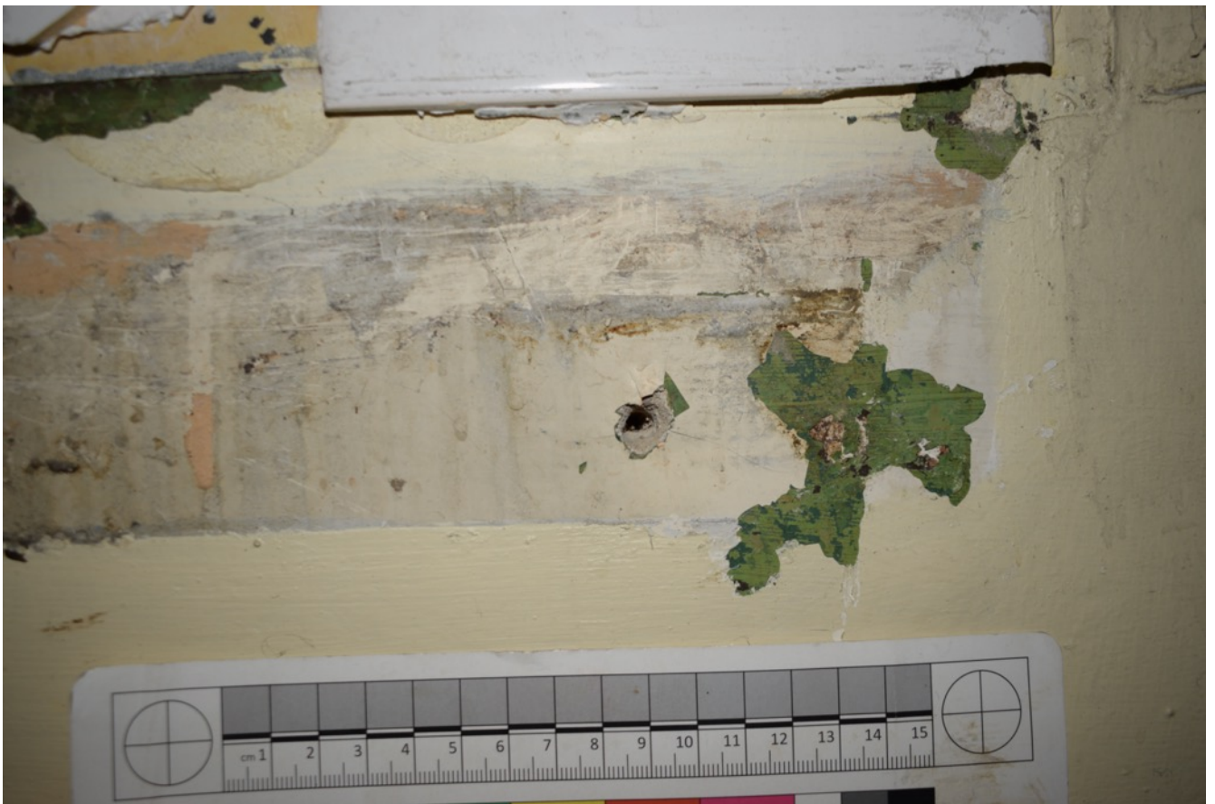
Figure 96: Evidence of colour scheme of the north-west anteroom at one stage (Author 2022).
