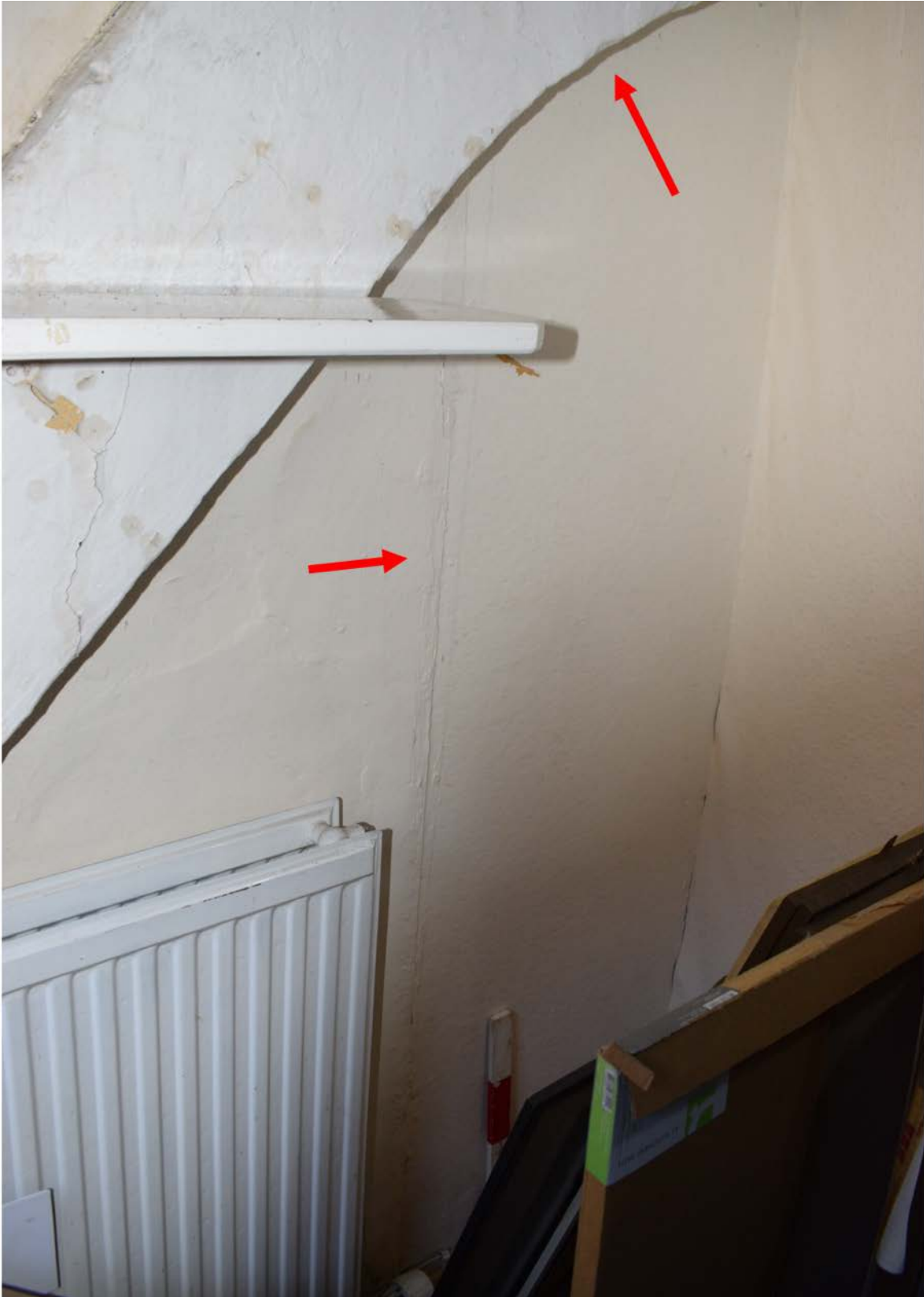
Figure 28: North wall of Room 49 showing blocked up doorway and diagonal beam. Room 49 no longer retains its original footprint (Author 2022).
