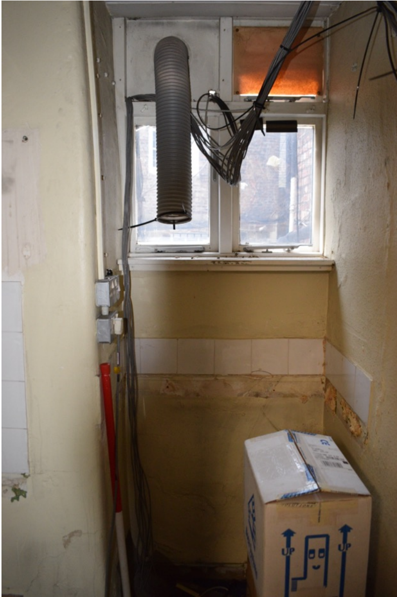
Figure 94: North-west anteroom off 1 st floor rear room facing west. This room was originally part of the 18 th century theatre passage. The window was the original location of the threshold that would have led into the TRY (Author 2022).
