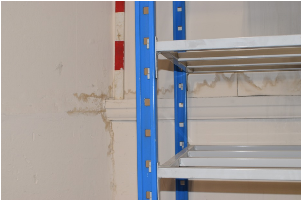
Figure 93: Evidence of dado rail on eastern wall of 1 st floor rear room (Author 2022).
