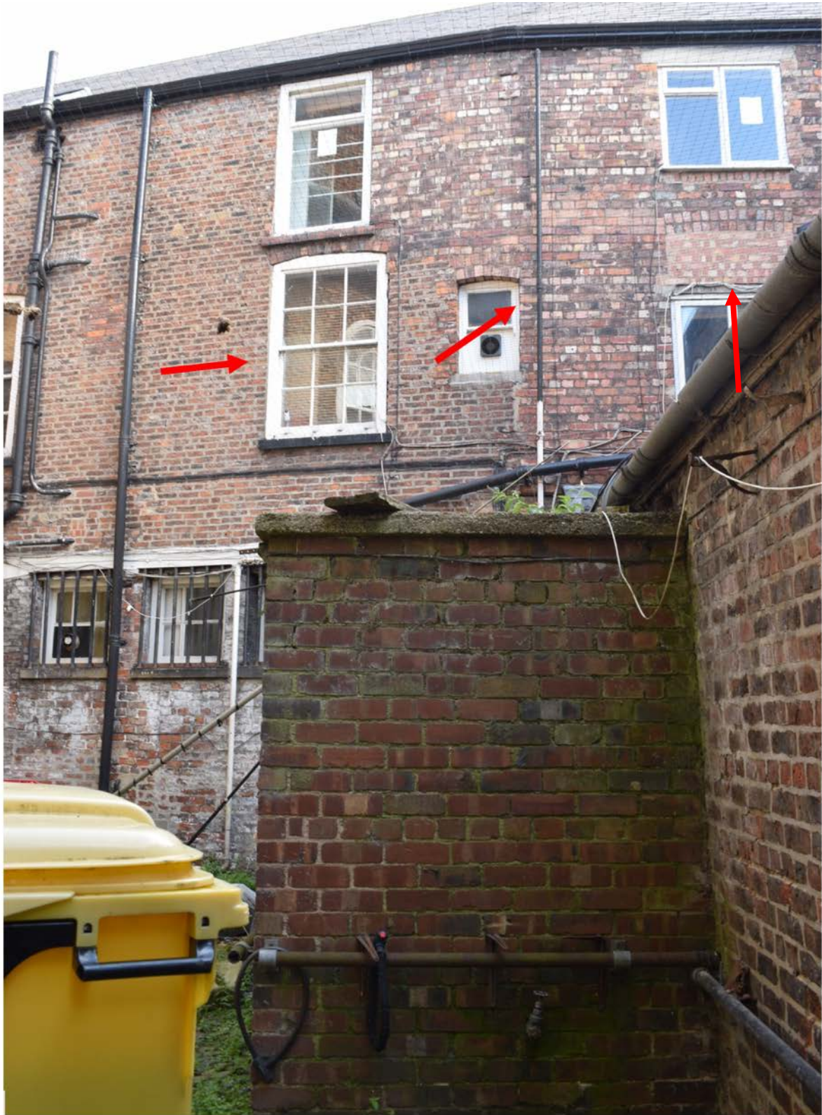
Figure 19: External south elevation of the TRY from the yard (18). Original sash window from Wilkinson's dressing room (22) on the left. Changes in brick work reveals where the wall has been rebuilt following the removal of the stage passage (21) on the right (Author 2022).
