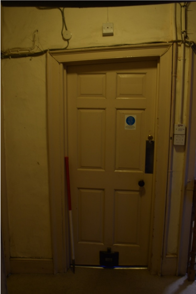
Figure 84: 1 st floor landing south facing door to former drawing room, now offices (Author 2022).
