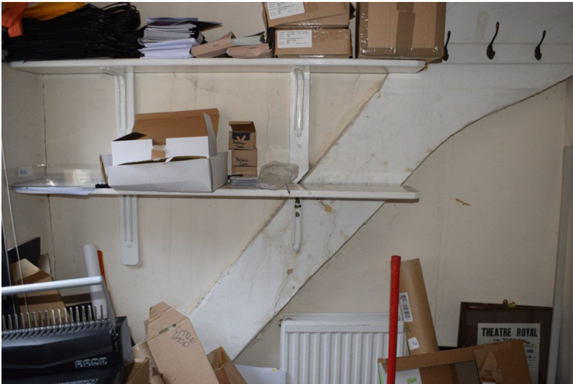
Figure 109: 2 nd floor western room facing north. In the east corner is the remains of a doorway (Author 2022).
