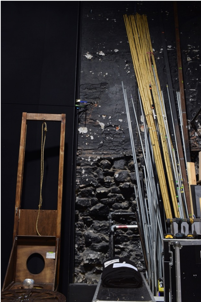
Figure 61: Internal east wall of theatre wing showing 1 st floor level line (Author 2022).
