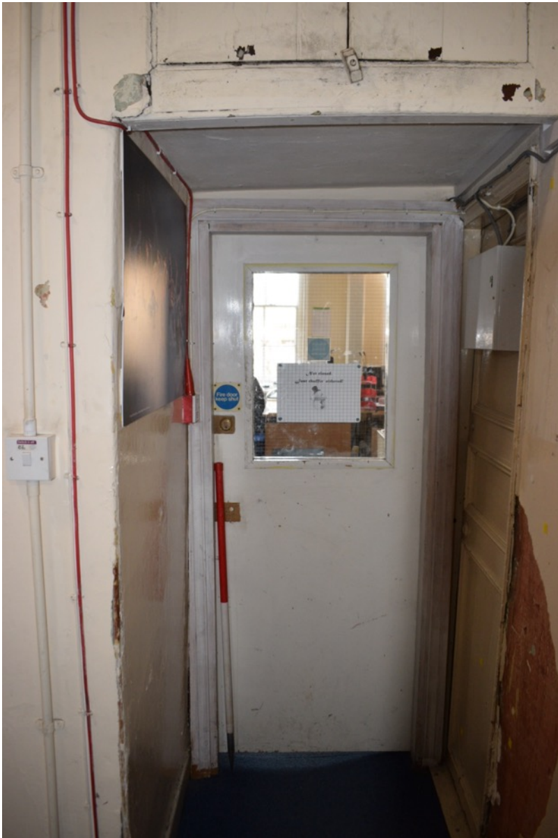
Figure 104: 2 nd floor landing looking south. Door leads to 2 nd floor front room (Author 2022).
