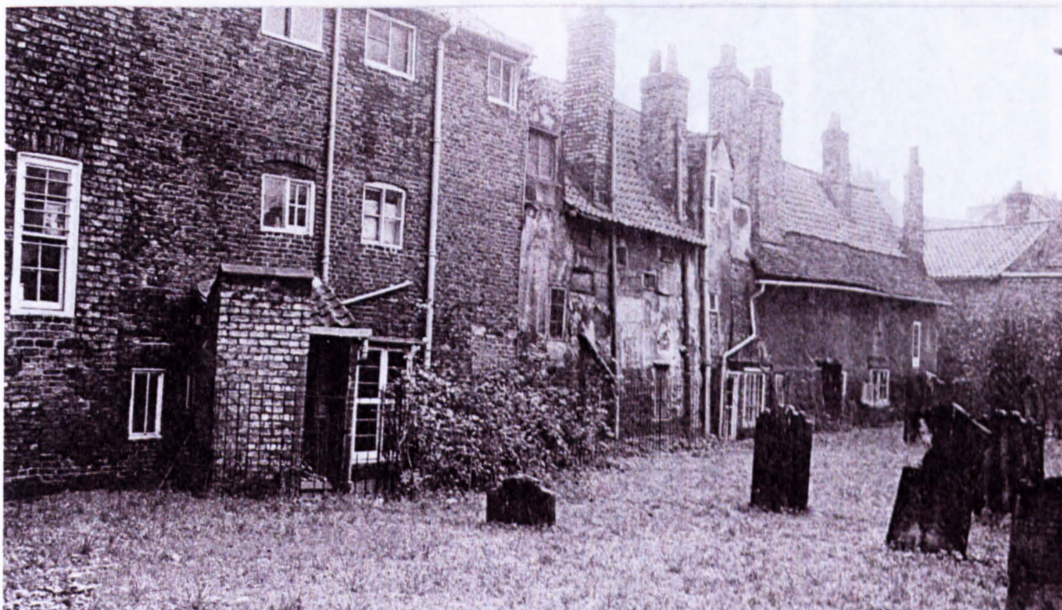
Fig. x Historic photograph (late C19th?) of the rear of the site, showing the brick lean-to prior to rebuilding (© Historic England).
